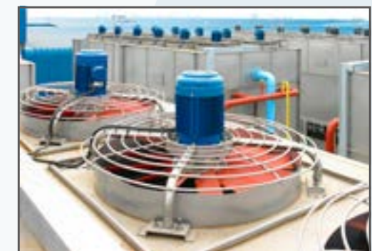
Fans and water pumps
